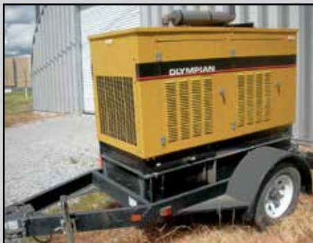
1998 CAT OLYMPIAN 20KVA GEN SET
