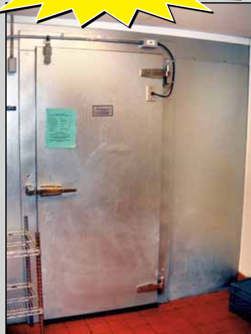
2006 REFRIGERATED STRUCTURE OF NEW ENGLAND WALK-IN FREEZER
